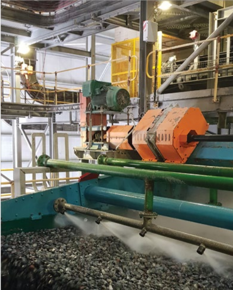
A WEG motor in a screening application.
