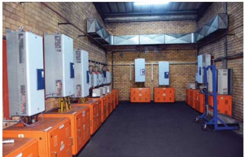
Wall mounted WEG CFW11 Variable Speed Drives with reactor cabinets on a mine site.
